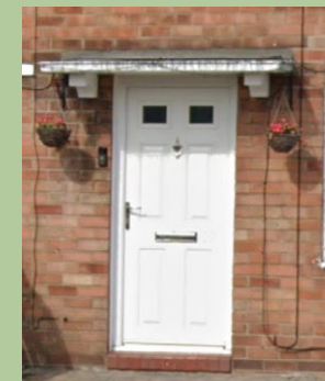
Composite door with flat canopy, present on most dwellings along Poplars Avenue.
